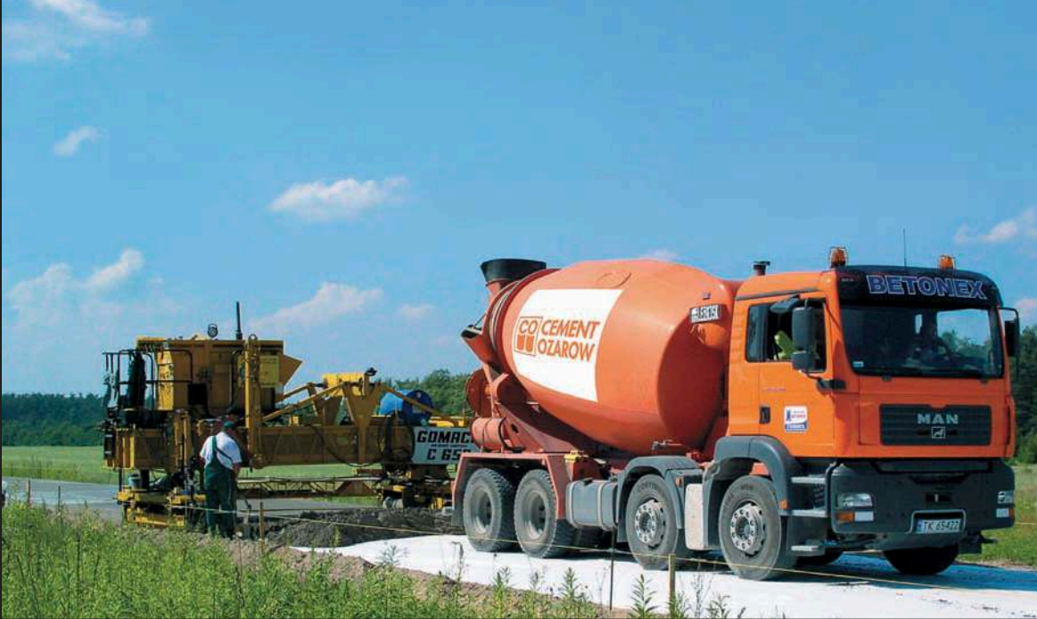
A section of a new six kilometre concrete road being laid by Grupa Ożarów for the town council in Ożarów. Concrete is seen increasingly as a cost-effective alternative for local roads in Poland.
